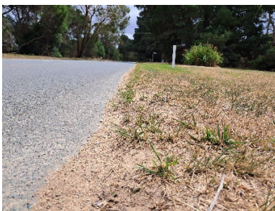
Subtle build up on edge of Merricks Beach Road, preventing flow into swale
