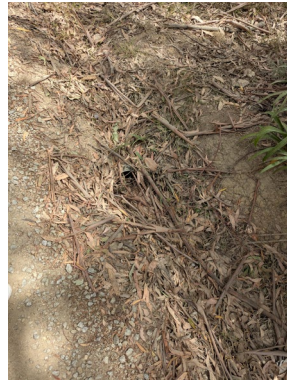
Crossover buried/not maintained
